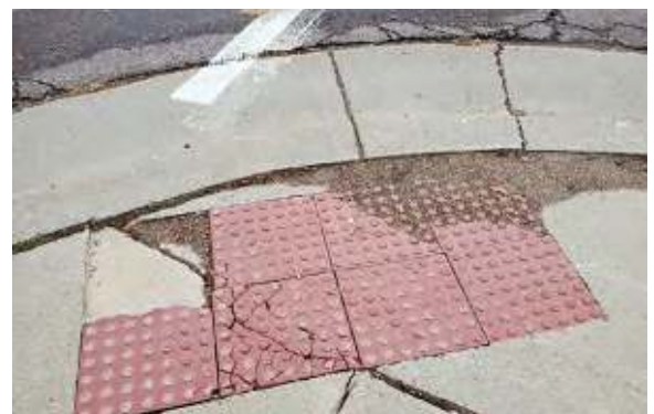
Infrastructure in need of maintenance
