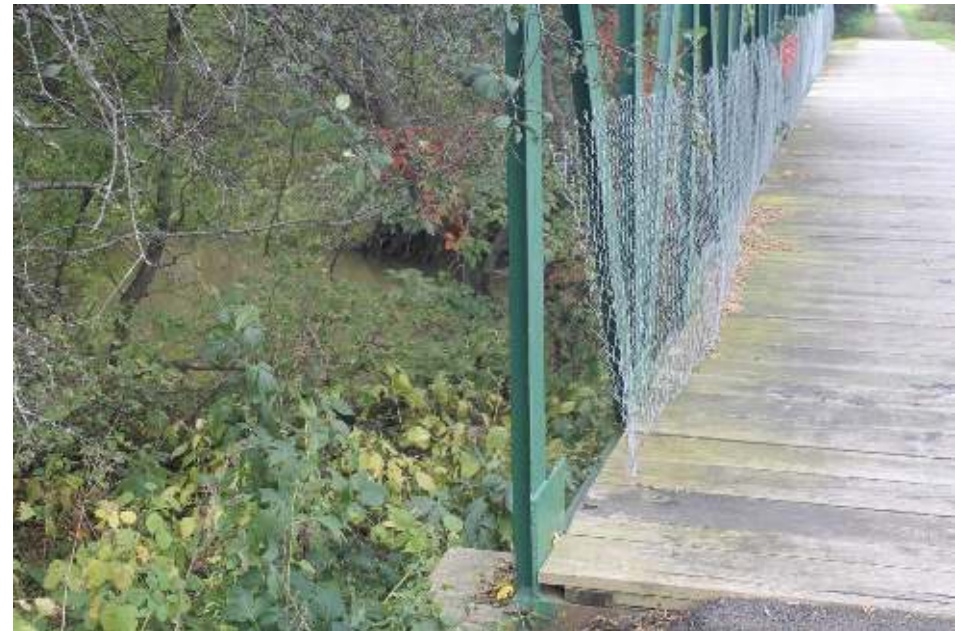
FIGURE 10: DETACHED FENCING ALONG THE WESTERN BRIDGE OF THE WALKING PATH
